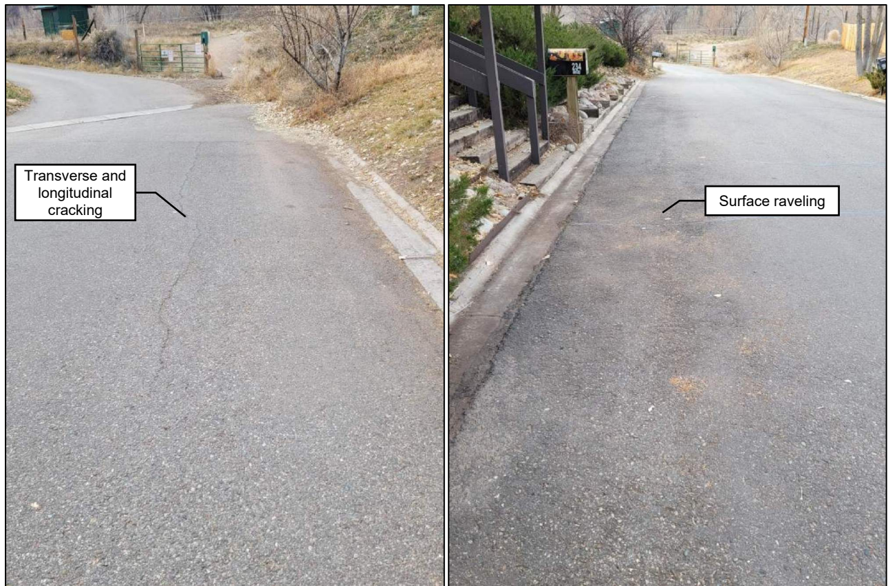
Figure 3-9. Yuma Roadway Conditions
